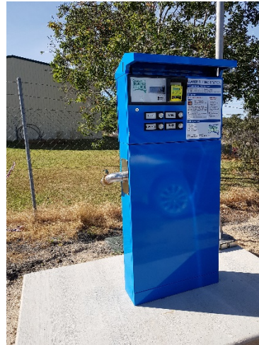
Texas Water Fill Station Flemming St, Texas
